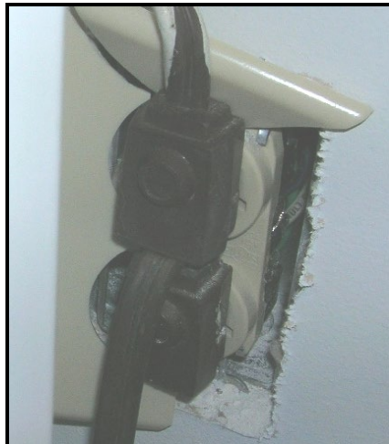
Figure 1-5.--Broken Cover Plate
