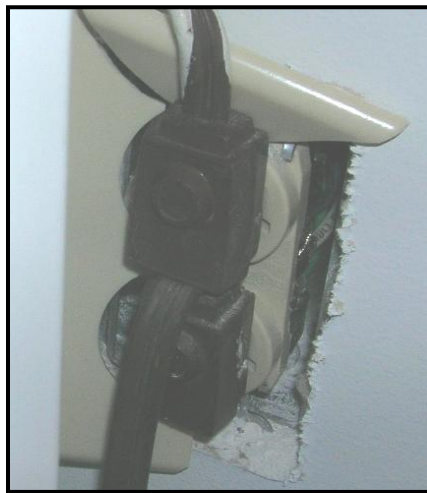
Figure 1-5.--Broken Cover Plate
